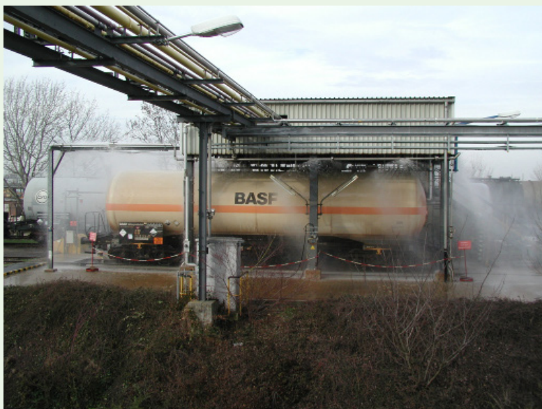
Figure 24 The ammonia loading area. The complete RTC is covered with water from the hydro-shields
